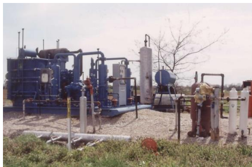
Compressor Station with Desiccant Dehydrator
